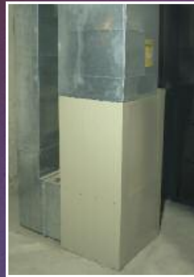
Hydro-air and heat pump backup
